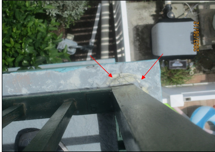
Photograph No. IMG_8660– Cracks in railing post pocket in landing of stairs adjacent to Unit 201.
