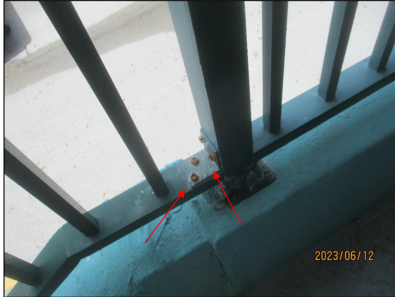
Photograph No. IMG_8641– Corroded metallic screws and bolts at the staircase railing adjacent to Unit 207.
