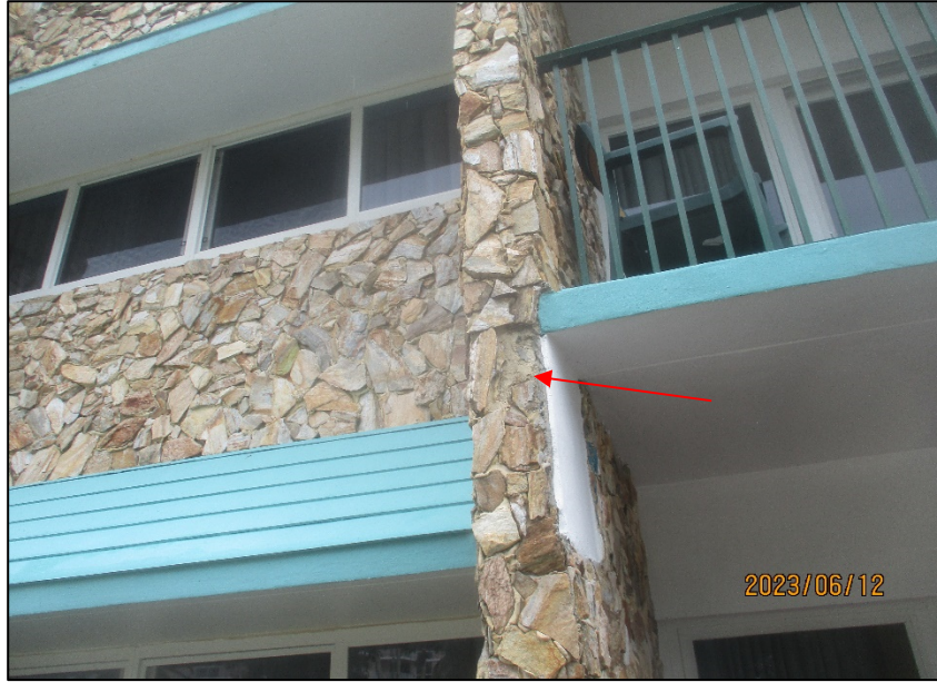
Photograph No. IMG_8580– Missing stone finishes adjacent to Unit 102, East Elevation – Level 1.
