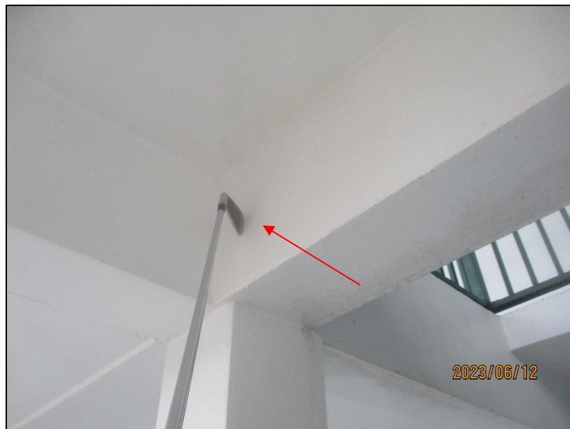
Photograph No. IMG_8610 – Delaminated stucco located at the beam adjacent to Unit 210 – Level 2 – Building Hallways.
