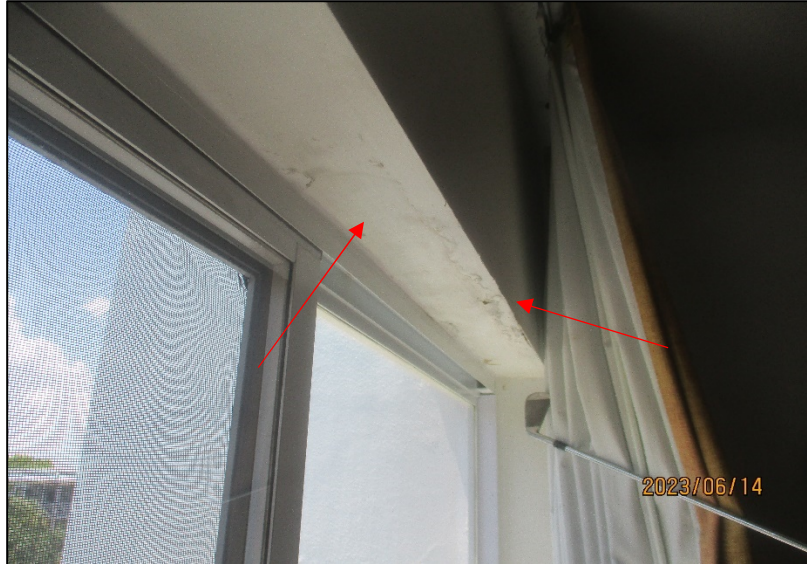
Photograph No. IMG_ 9035– Signs of water infiltration at the interior window in Unit 312- Level 3.
