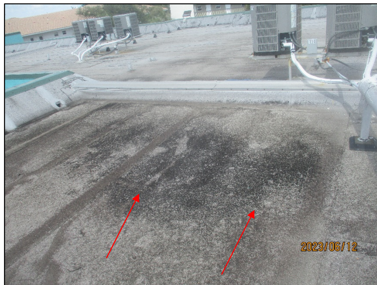
Photograph No. IMG_8503 – Signs of water ponding located at Southwest wing of the building roof.
