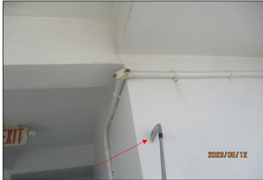
Photograph No. IMG_8649 – Delaminated stucco located at the exterior wall corner of Unit 204 – Level 2 – Building Hallways.
