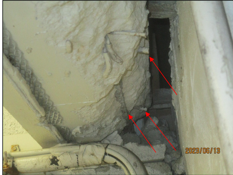
Photograph No. IMG_8751 – Exposed rebar at storage ceiling, located adjacent to Unit 204 at the 2 nd level.
