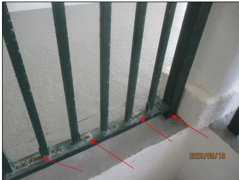
Photograph No. IMG_8828– Corroded screws and bolts at the staircase railings adjacent to Unit 211 – Level 2.
