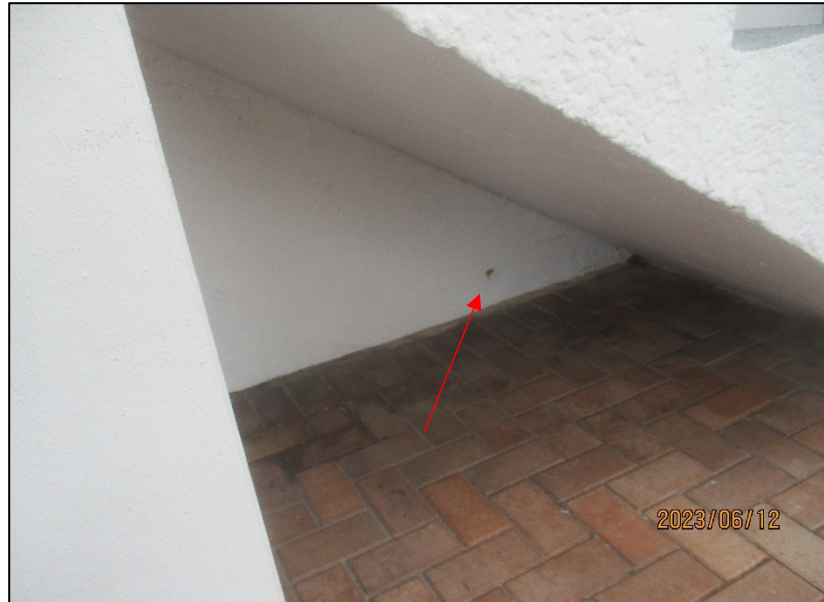
Photograph No. IMG_8568– Corrosion stain below the staircase that is adjacent to Unit 103.
