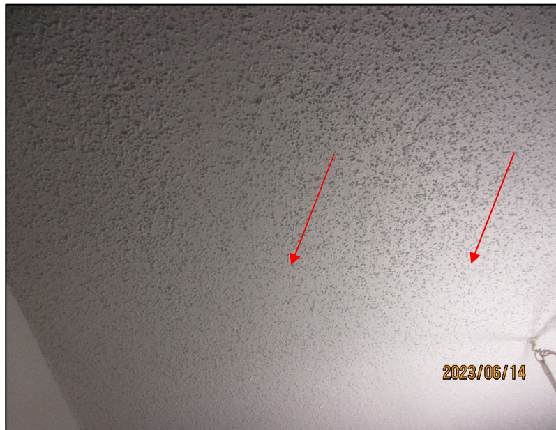
Photograph No. IMG_9030 – Overhead interior ceiling crack at the living room of Unit 312 on the 3 rd level.
