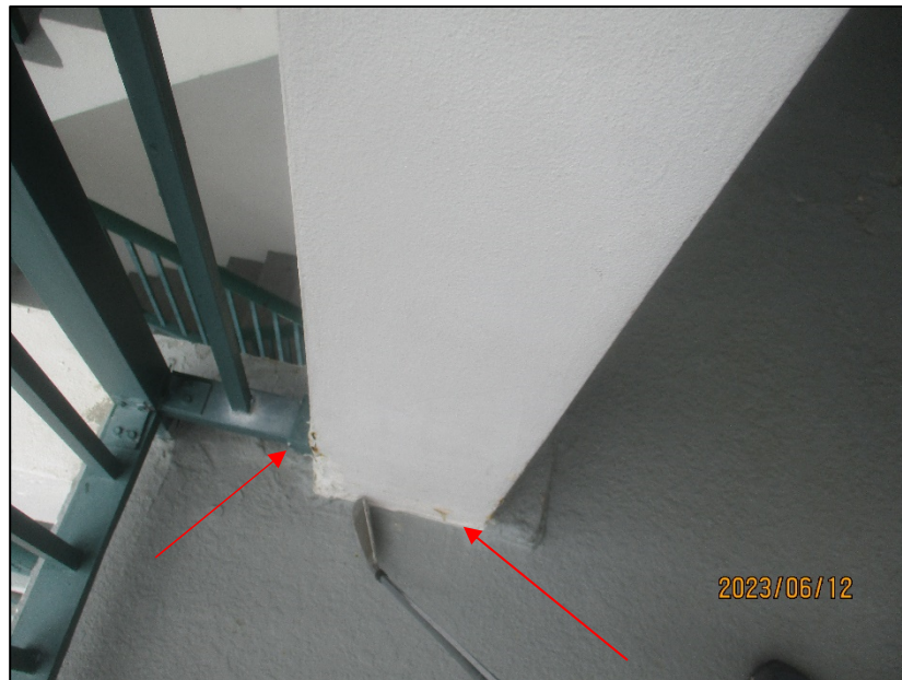
Photograph No. IMG_8670– Corrosion stains at the column adjacent to the stairs near Unit 303, 3 rd level.
