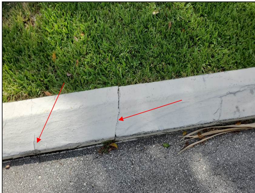
Photograph No. IMG_20230612-100939– Cracks in the concrete curb located adjacent to the planter in front of the main entrance of the building.
