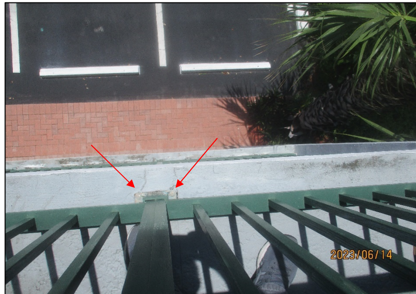
Photograph No. IMG_9041– Cracks in balcony railing post pocket of Unit 311 – Level 3.
