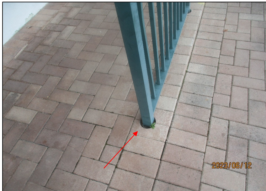
Photograph No. IMG_8560 – Depressed railing post pocket in front of Unit 105 -Level 1.
