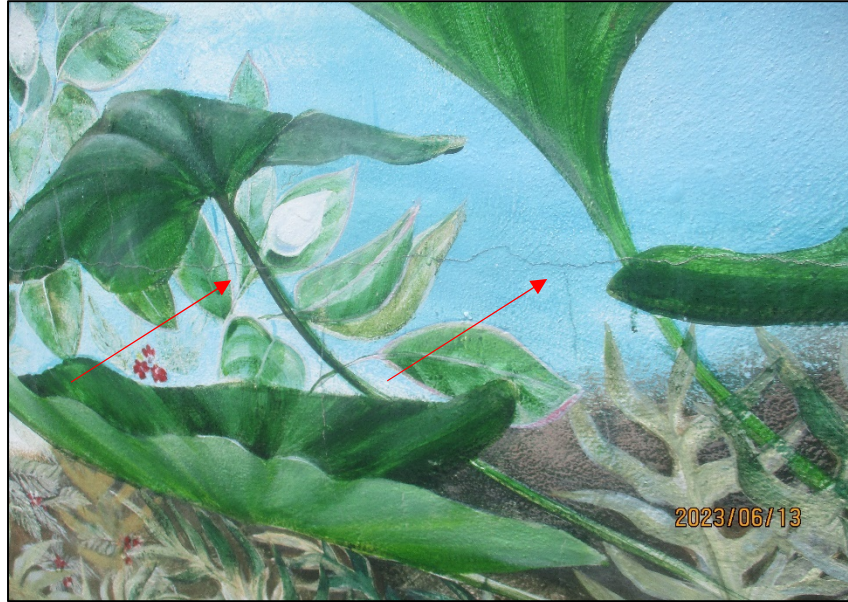
Photograph No. IMG_8770 – Stucco cracks located on the artistic painting wall on the South Elevation near the pool deck.
