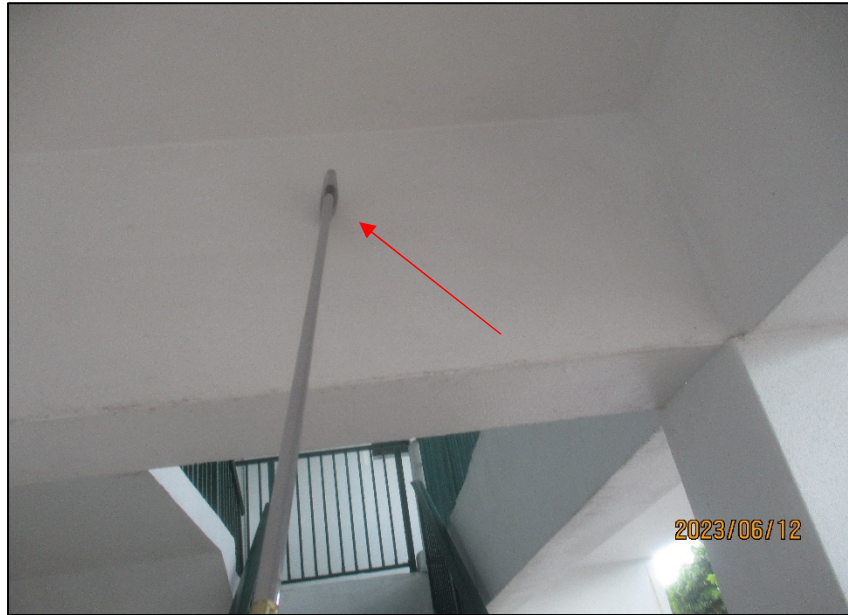
Photograph No. IMG_8527 – Delaminated stucco located at the beam adjacent to Unit 110 - Level 1- Building Hallways.
