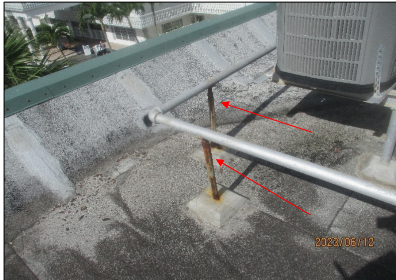
Photograph No. IMG_8469 – Gas pipe metallic supports are corroded at the East wing - Building Roof.
