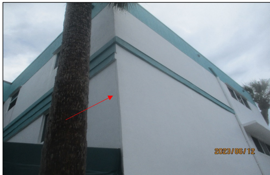
Photograph No. IMG_8598 – Stucco crack located at the West Elevation wall corner adjacent to the South Elevation.
