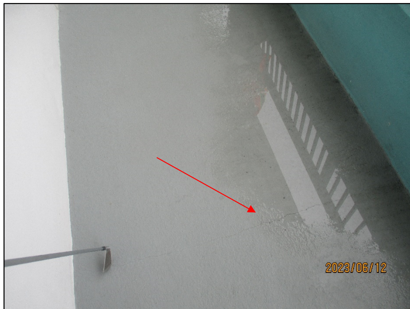
Photograph No.IMG_8708 – Crack in hallway floor slab in front of Unit 316 at the 3 rd level.
