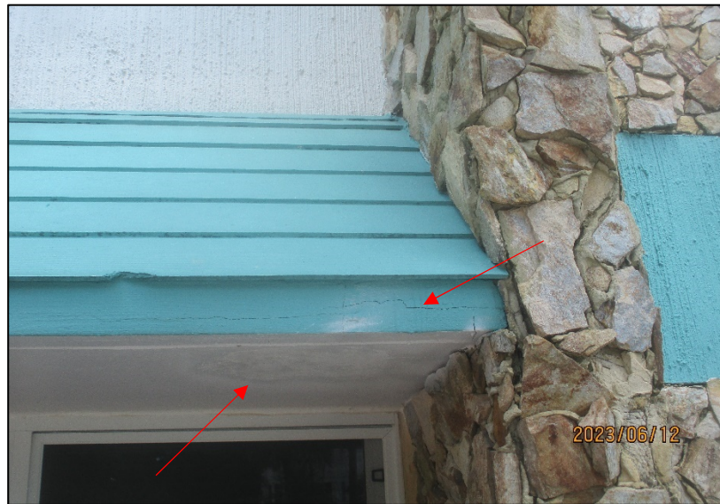
Photograph No. IMG_ 8576– Signs of water infiltration at the ceiling slab over the exterior window of the Administration Office – East Elevation.
