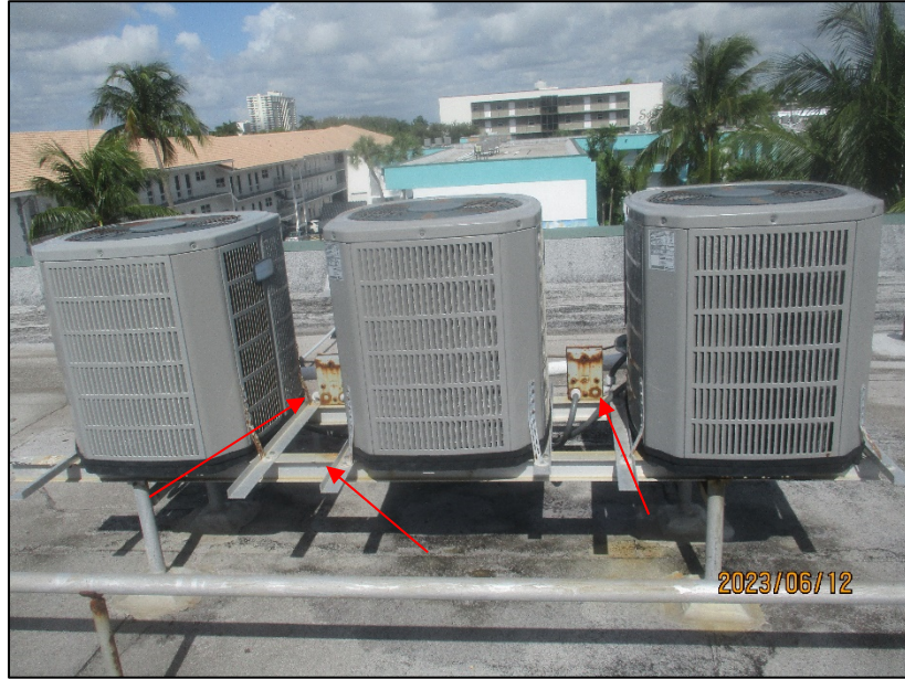
Photograph No. IMG_8478– Corroded metallic components of the A/C equipment - Building Roof.
