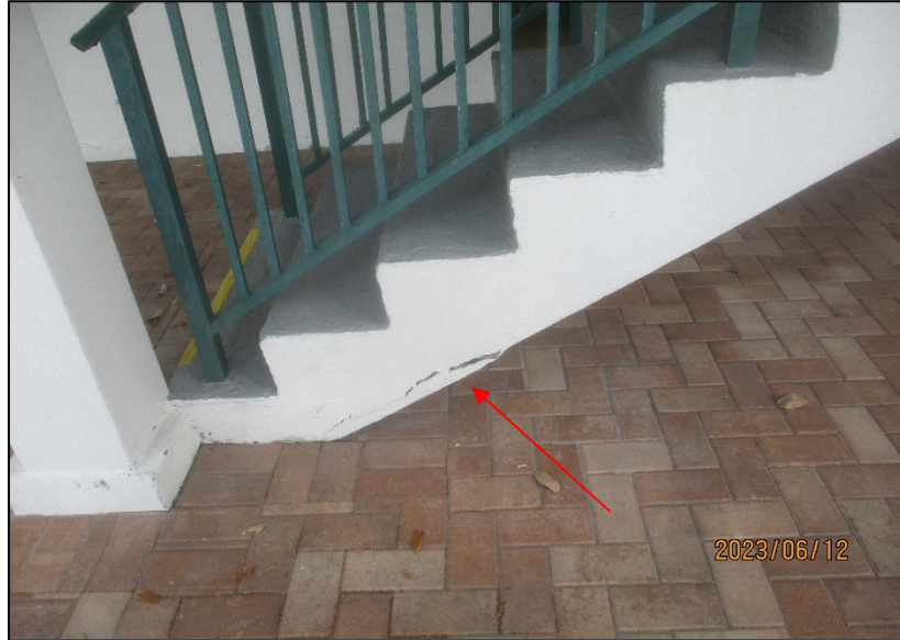
Photograph No. IMG_8532 – Delaminated/spalled concrete at the underside of the staircase adjacent to Unit 110 at the 1 st level.
