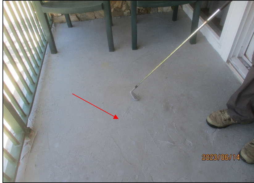
Photograph No. IMG_9075 – Delaminated concrete at balcony floor slab of Unit 302 at the 3 rd level.
