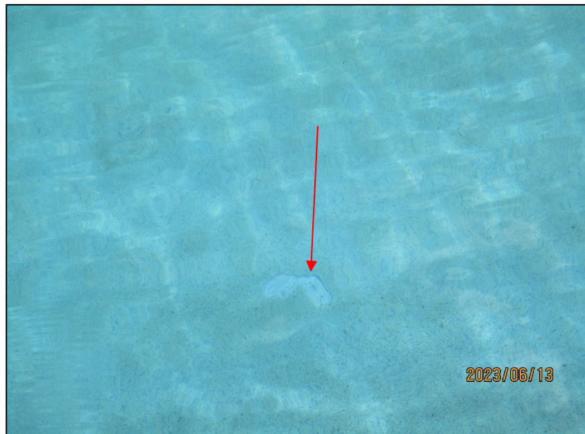
Photograph No. IMG_8777– Missing finishes at North side of the Pool near the pool stairs.
