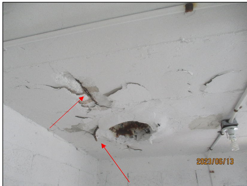
Photograph No. IMG_8736 – Concrete spalling/exposed rebar at the ceiling slab of the Pool Room.
