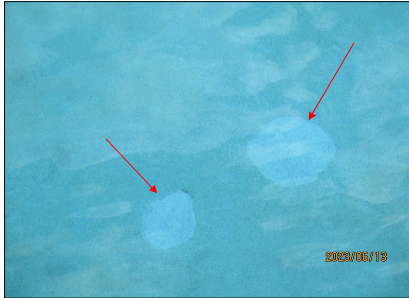
Photograph No. IMG_8776– Missing finishes at South side of the Pool near the white fence.
