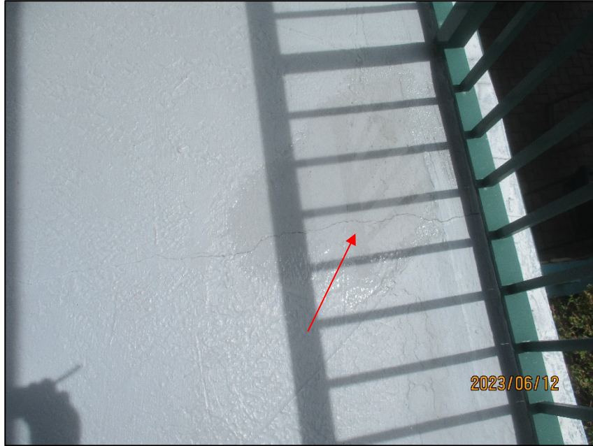
Photograph No. IMG_8654 – Crack in hallway floor slab in front of Unit 201 at the 2 nd level.
