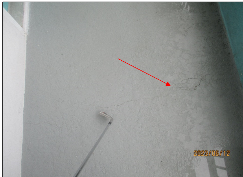
Photograph No.IMG_8707 – Delaminated concrete at the hallway floor slab in front of Unit 315.
