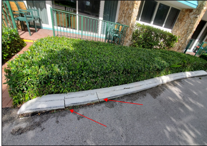
Photograph No. IMG_20230612-101541– Multiple cracks/debonded concrete in the concrete curb in front of Unit 101 – East side of the building.
