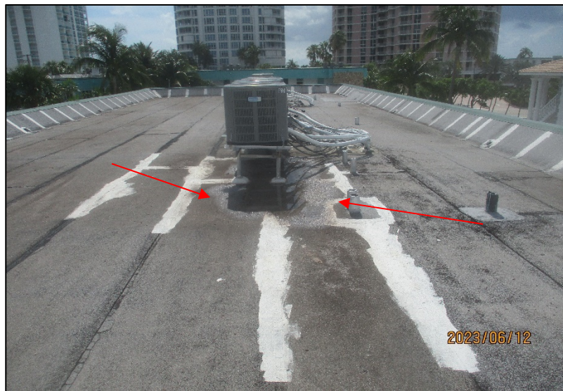
Photograph No. IMG_8511 – Signs of water ponding below the A/C equipment at the South wing of the building roof.
