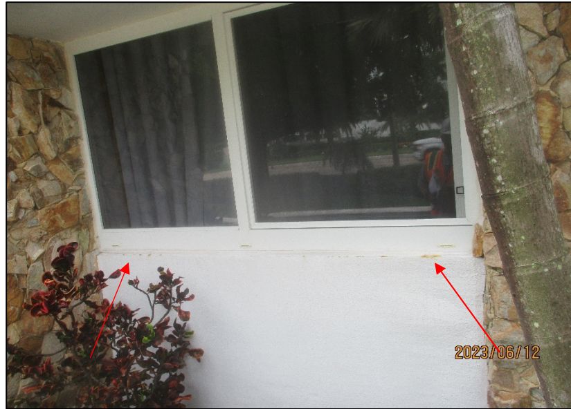
Photograph No. IMG_8579– Corrosion stain at the exterior window sill of the Administration Office, East Elevation.
