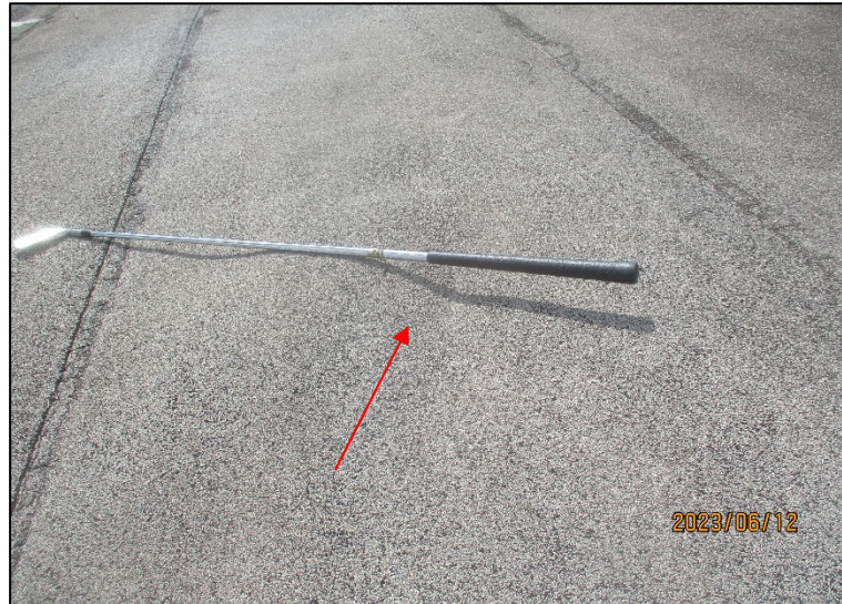
Photograph No. IMG_8516 – Air/water blisters under the building roofing membrane located at the Southwest wing of the building roof.
